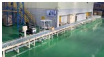
E Plant : E-Beam Irradiation Facility
